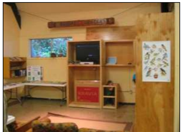
The new cabinets in the lodge take shape. They will house the 32" LCD TV with VCR and DVD player donated by Bruce Flaming.
